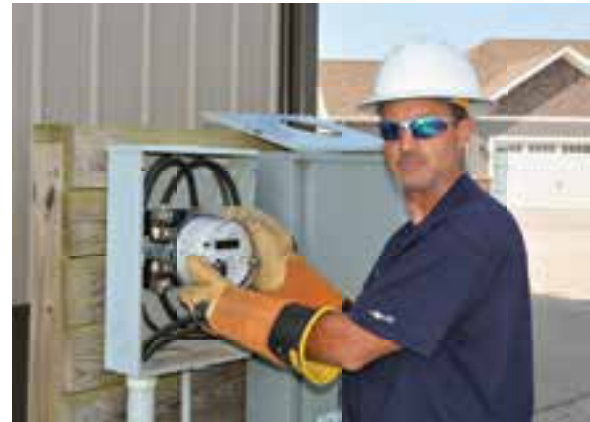
EnerStar has started beta testing the new meters that will be installed at all account locations over the next year. Here, EnerStar's Chad Cornwell switches one of the first meters deployed. The current electric meters in use were installed in 2010.
